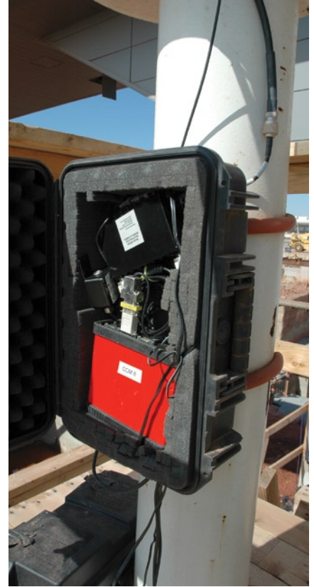
Radio modem enclosure made from off-the-shelf watertight plastic gun case.
