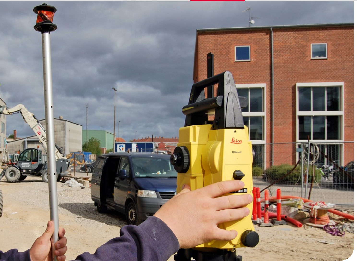
■ Jonas Nielsen finishing a subcontractor job preparing the terrain for a large house-building project.
