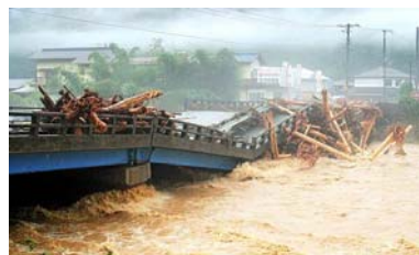
Torrential rains and severe flooding.
