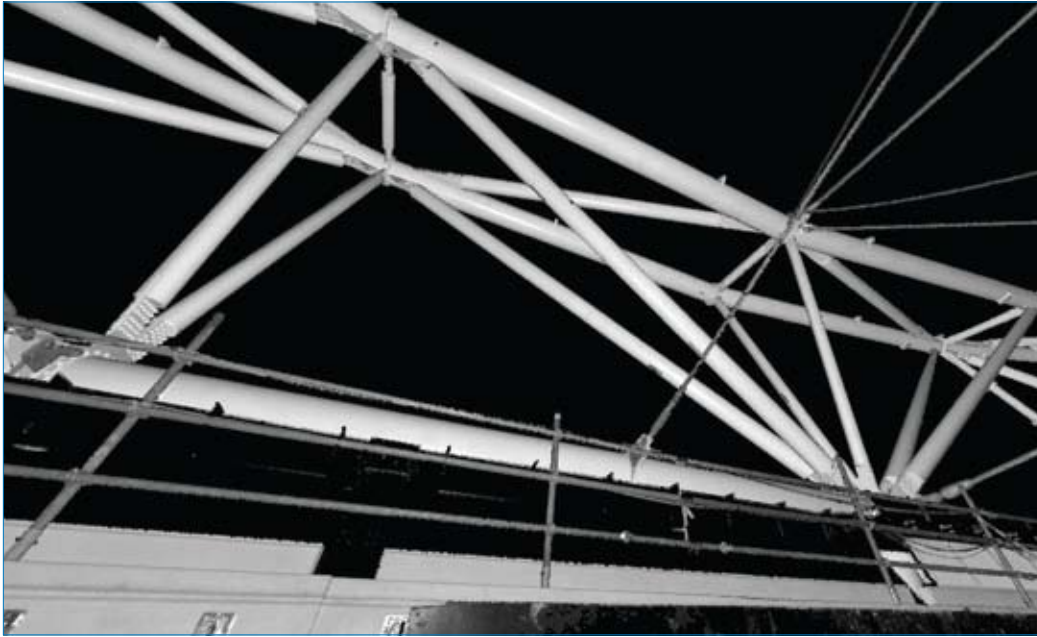
This high-resolution scan of the roof-supporting structure was taken using a high-speed phase-based 3D laser scanner. The point cloud is displayed in grey-scale intensity mapping, with locating holes and individual rivets visible.
